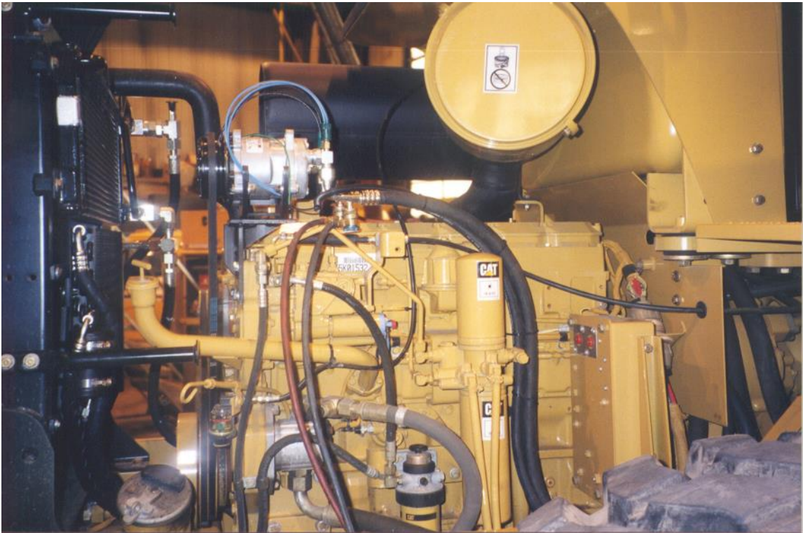
Compressor in place showing line runs.
